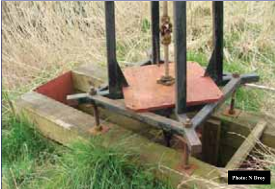
Fig 5: Sail unit is secured to pumping chamber
