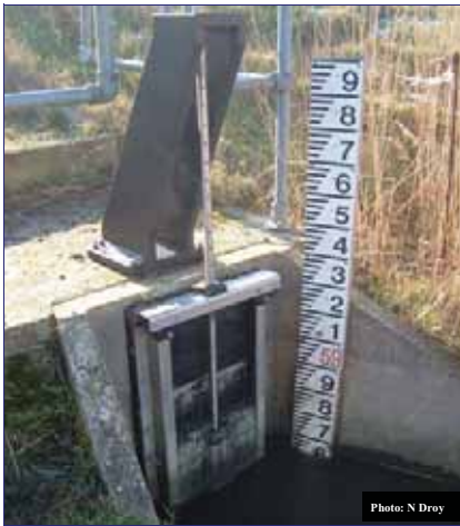
Fig 1: Penstock weir & gauge board
