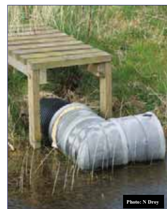
Fig 7: Right angled bend (& operator access platform)
