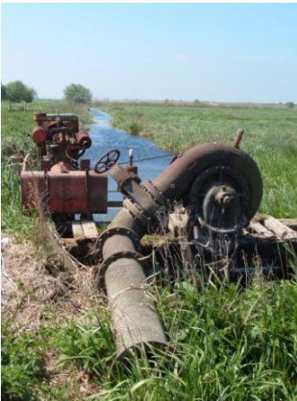
Pump infrastructure, Cambs.
