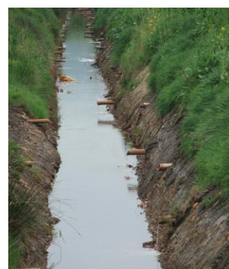
Drainage outfall pipes from successive schemes, Yorks. Note the differing levels of pipes.
