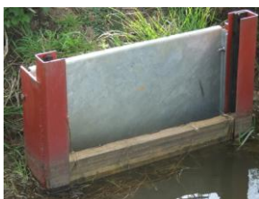
Drop board sluice
